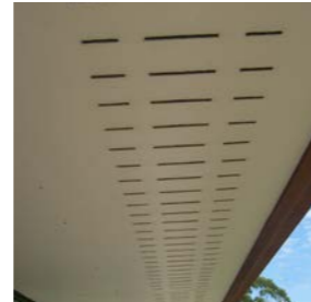
Slotted Hardiflex soffit sheeting
